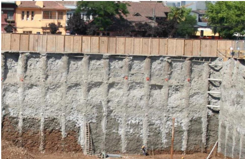
Figure 1. Retaining wall using discontinuous and anchored bored piles. Source: Pilotes Terratest, n.d.a.
