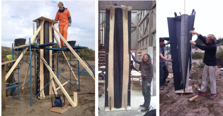
The formworks stands as an independent body that is fixed to the ground before concrete pouring takes place. Later, once the concrete has hardened, the geotextile and ply formwork is taken apart.
