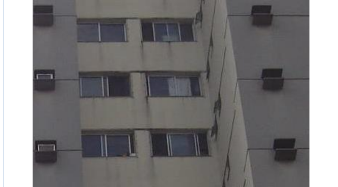
Fig. 8: Stains formed close to windowsill of Building 5. Facade W (Developed by the authors)
