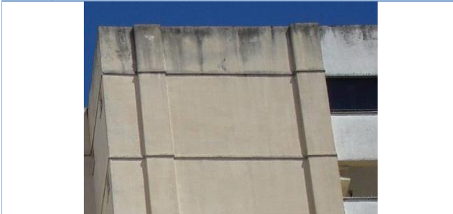
Fig. 7: Stains formed in platbands of Building 3. Facade N (Developed by the authors).
