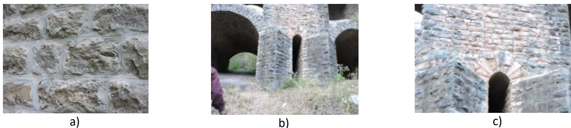
Figure 2. Present condition of Bridge No. 541, Kalka Shimla mountain railways: a) patches on the pier; b) bottom piers covered with the soil; c) efflorescence. (Self-Elaboration).
