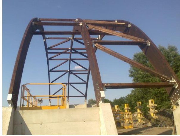
Figure 1. Construction of truss-braced timber arches of a sport hall in Hungary. Source: Self-Elaboration.
