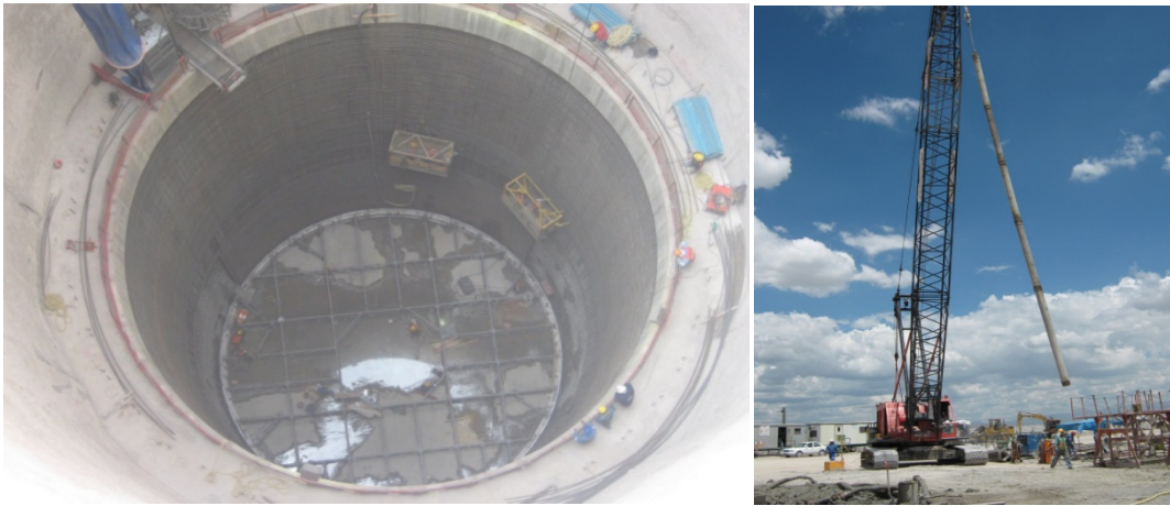
Figure 6. Structure for the bottom slab (left) and Installation of the pipeline to pour the concrete (right)
